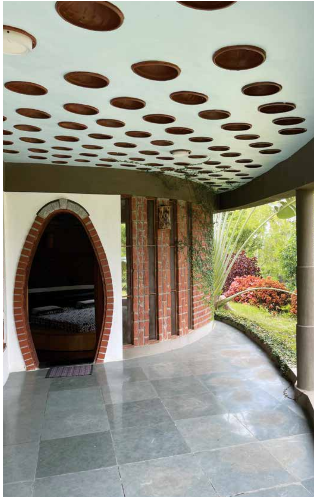
Unconventional egg shaped entry with filler slab concrete roof using custom made clay pots.
